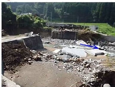
② 橋梁被災(流失)状況(小園橋)
